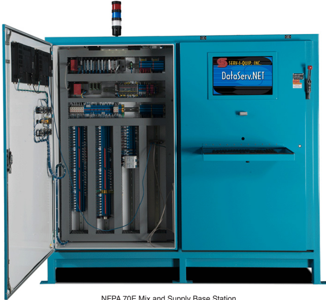
NFWA 70E Mix and Supply Base Station
